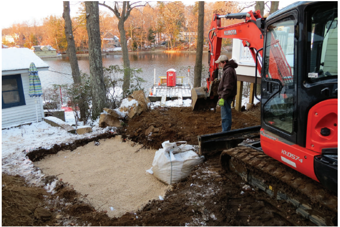
Avery Jinks of Septic Experts prepares to spread 3/4-inch crushed stone over the sand for the absorption bed. Some 20 feet below him is the barge with a portable sanitation unit.
