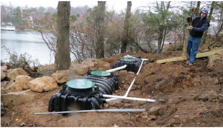
Bill Post of Septic Experts rolls up the rigging strap used to lift components and materials.
