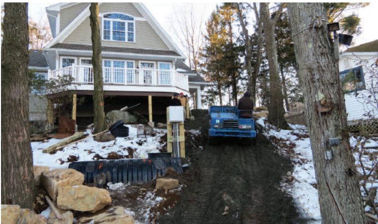
Avery Jinks of Septic Experts eases the IHI 1.3-cubic-yard IC30 crawler carrier up the steep slope past the septic tank and control panel to deliver another load of bank run.
