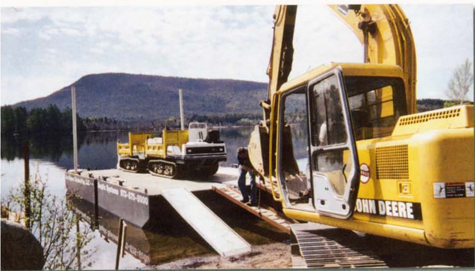
On the deck of the barge are two rubber tracked dumps to haul material around island.
