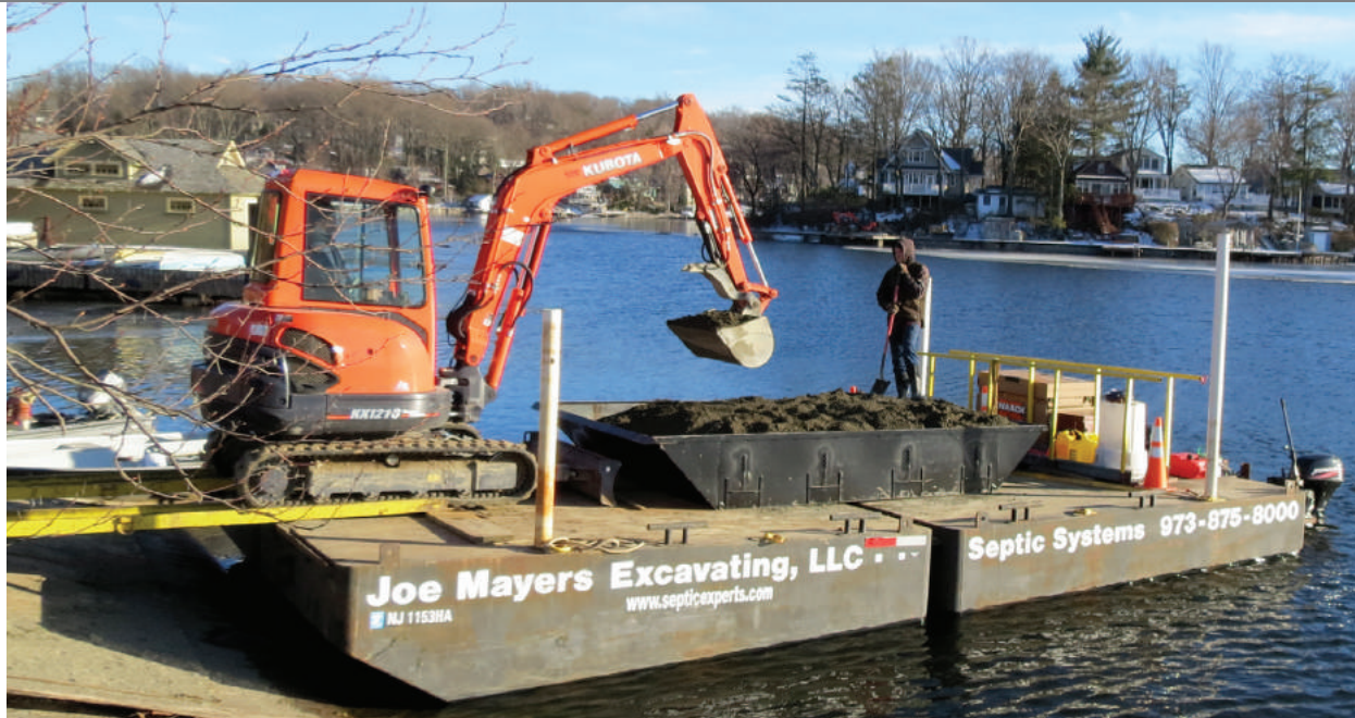
Using a Kubota 121 excavator, Bill Post of Septic Experts places screened fill in a 14- by 7- by 2-foot-high containment pan on a barge for transport to Raccoon Island. (Photos courtesy of Septic Experts)
